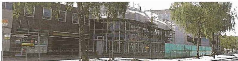
■ The former Riley's building which is being demolished to make way for Birketts
